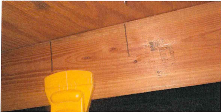
Nail location verified
